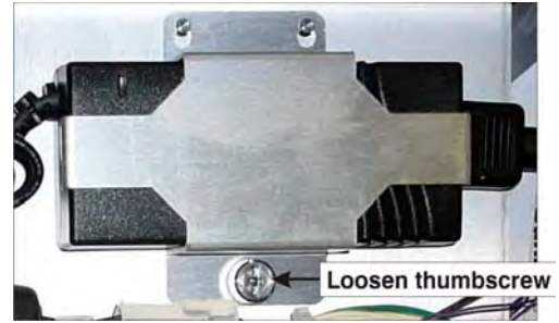
Figure 5-49 Standby Power Supply
